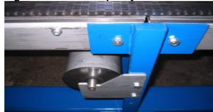
Figure 4. Belt return pulley
